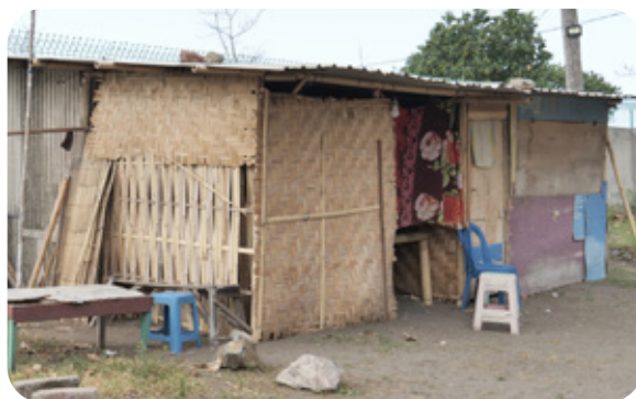
Original dilapidated house of orphan/poor family in Indonesia (source: IR Digital)
